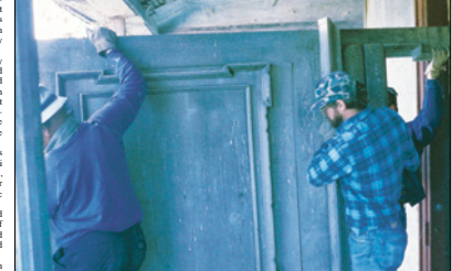
Woodwork being removed from Lyells to go to Bacon's Castle. Photo: Menokin
